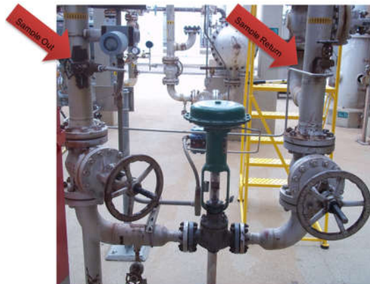
Typical sample taken across a control valve
