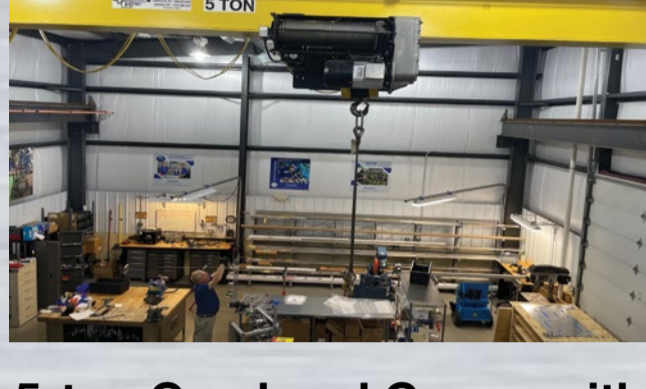
5-ton Overhead Crane, with 18-foot clearance
