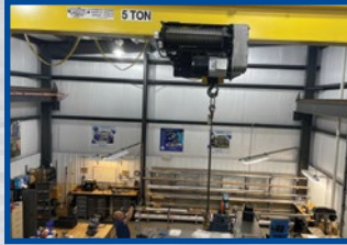
5-ton Overhead Crane, with 18-foot clearance
